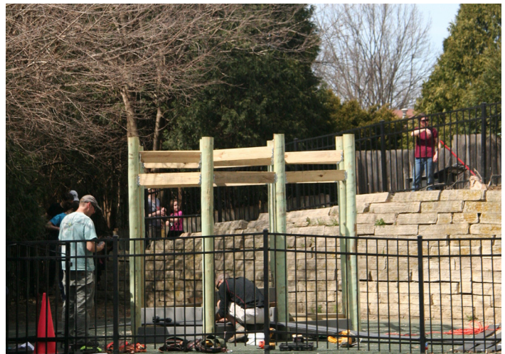
Parents building the new climbing and play structure on the preschool playground.
